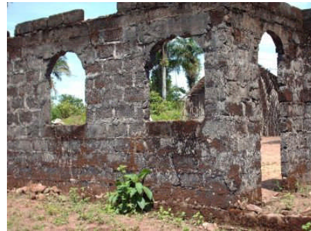
New church without roof or floor started 15 years ago
